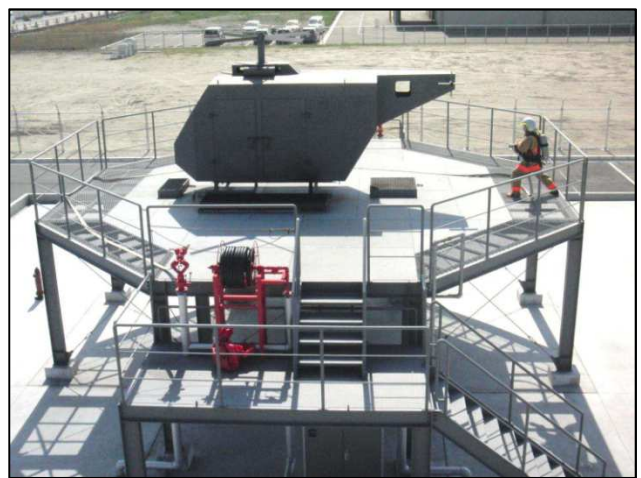
Fig.12 Heli-deck firefighting module
